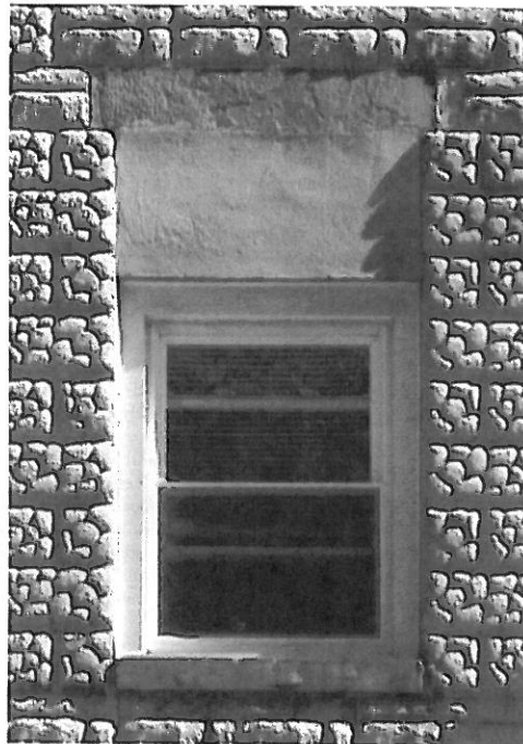
This window replacement resulted in reduced visibility and daylight.
